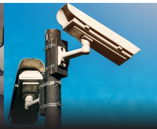
CCTV SURVEILLANCE AND SECURITY
